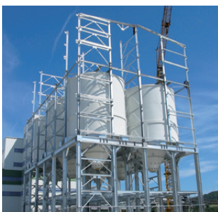
Sand drying and transportation, Provodín, Czech Republic Design office: CAB minerals s.r.o., Brno, Czech Republic
